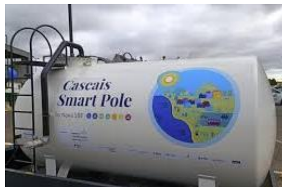
Biodiesel Storage Tank
